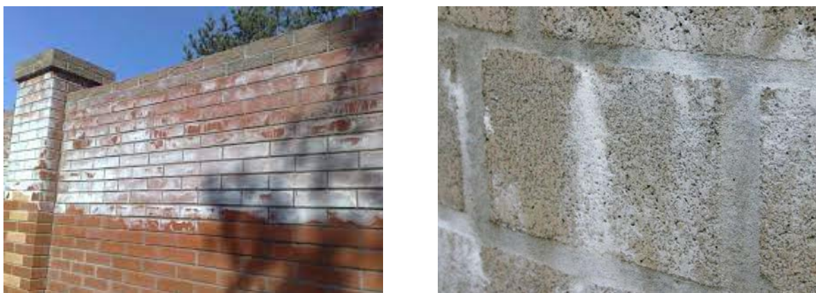
Figure 4. Examples of efflorescence's on brick and concrete masonry surfaces.
