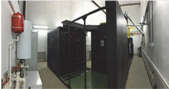
Fig. 1. Hydrogen plasma plant for the processing of industrial liquid waste
